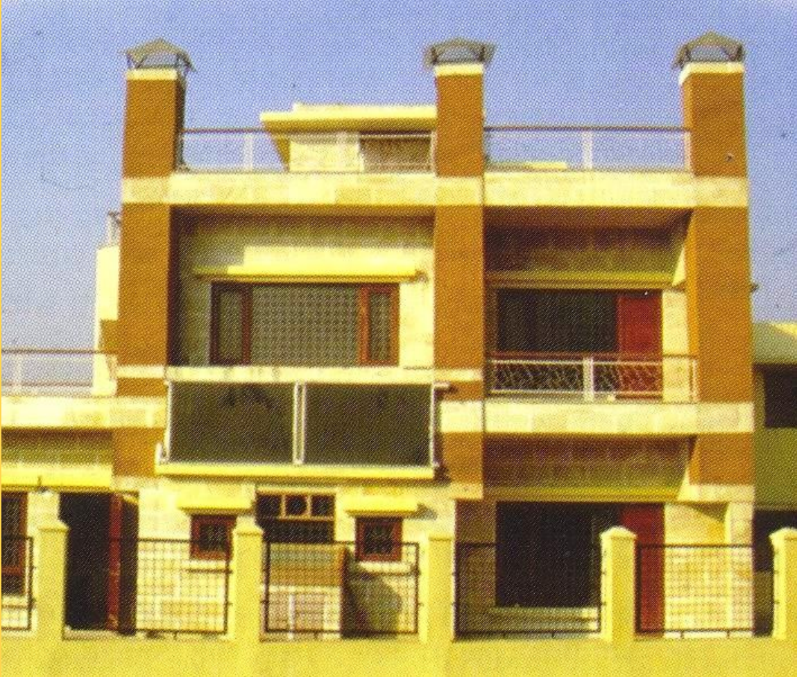
Fig. 6.3 Solar hot water systems in Sudha and Atam Kumar's residence in New Delhi [2]
