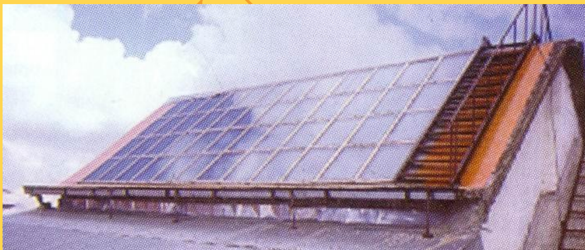
Fig.6.7 Photograph of solar air heating system at the HP State Co-operative Bank, Shimla [2]
